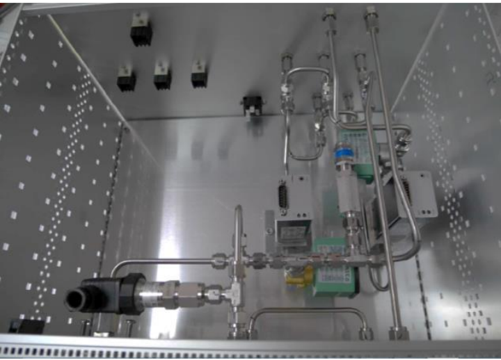
Inner part of the main gas rack
