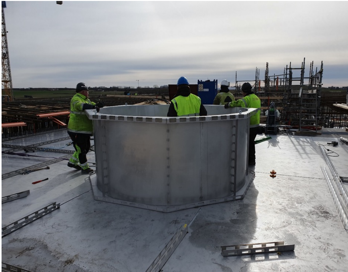
Confinement penetration in Process Cell ceiling
