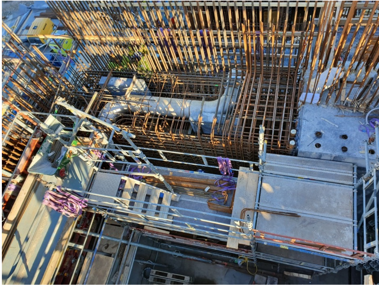
Process Cell ceiling start of HB slab rebar installation on top of liner plates
