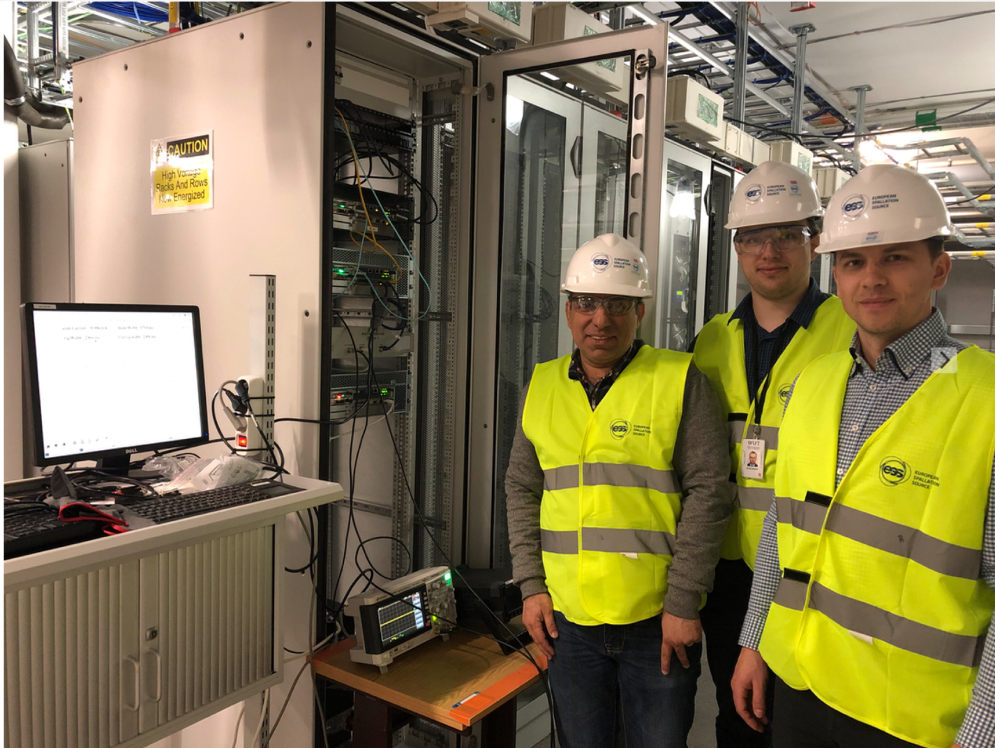
Delivery of the BCM electronics by WUT and site installation of the first AIU (10 April 2019)
