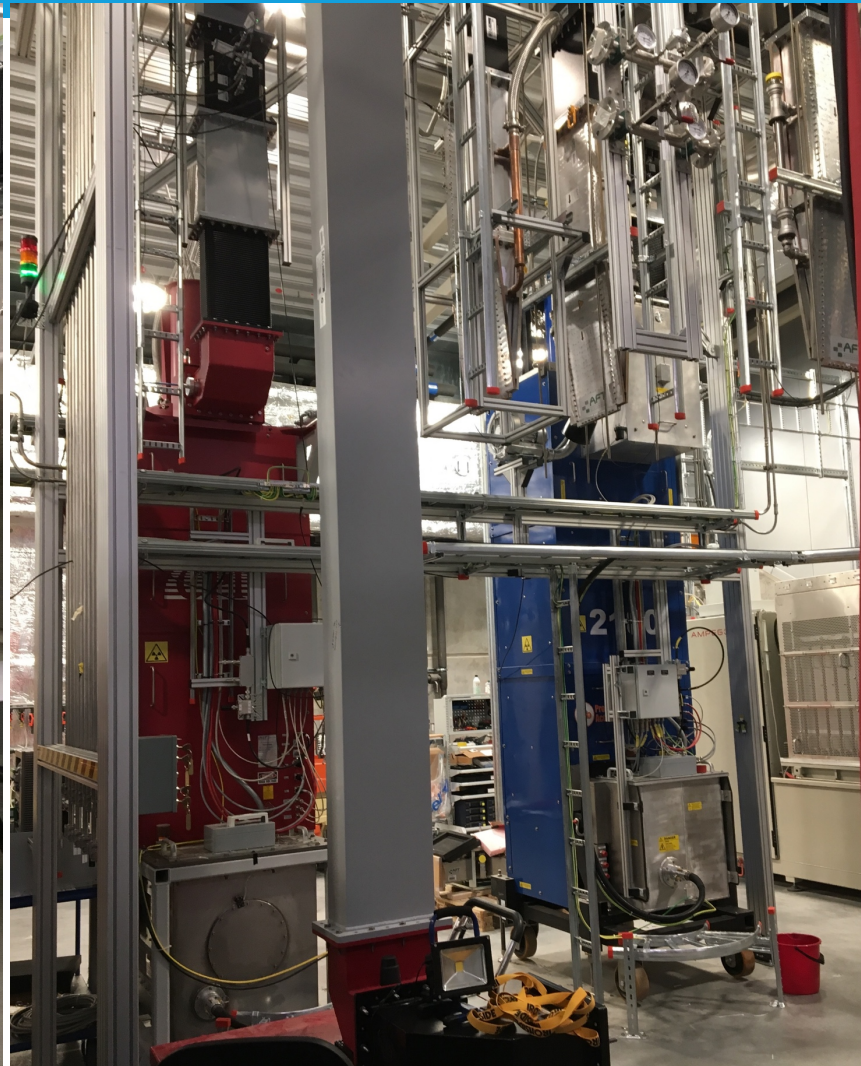
Klystron commissioning on loads
