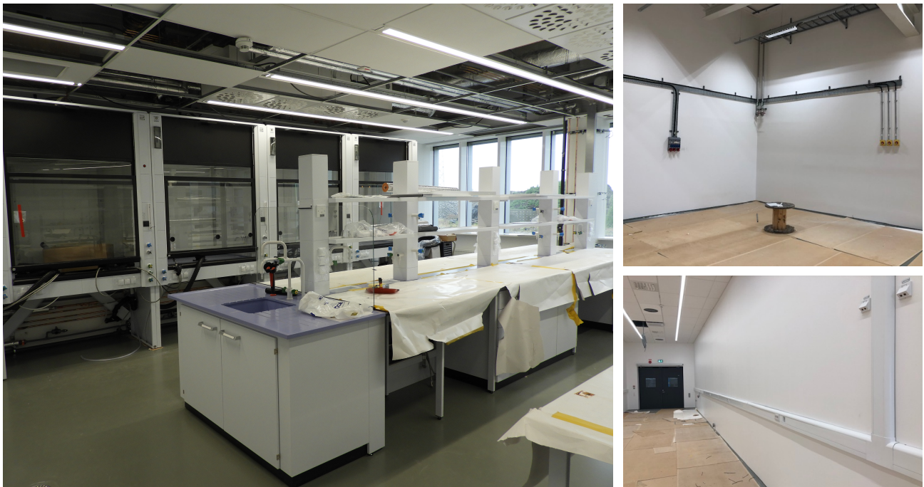
Figure 9: Physical Characterization lab 90% done (left). Electrical installation in technical laboratories (right – top: sample environment workshop, bottom: optics lab)
