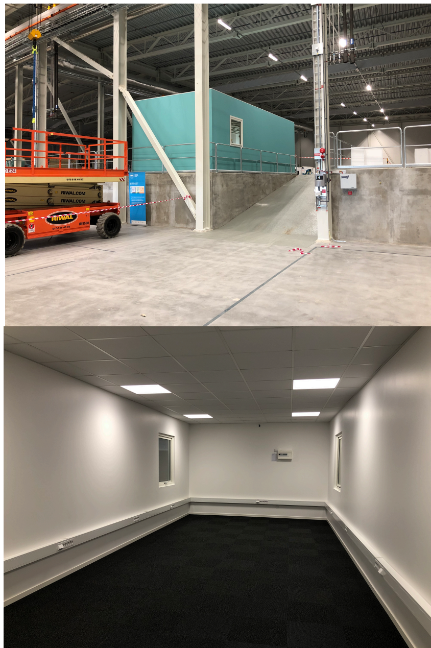
Figure 8 – Final product in position (top) and internally with all electrical circuits and lighting (bottom)
