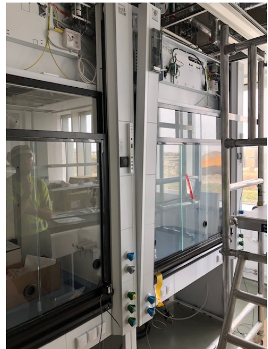
Figure 10: Chemical fume hoods testing with Siemens (building control system) and Sanber (fume hood/ducting specialist)
