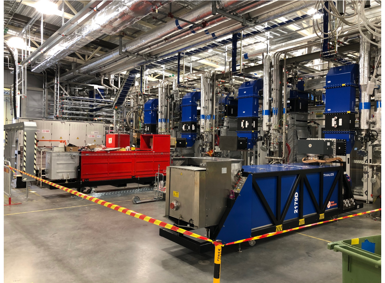
First Spoke RF station at TS3, already operating at 350 kW All of MB waveguide runs have been tuned, DTL4 & 5 in Gallery Electrical installation (cable pulling) started in SPK and MBL
