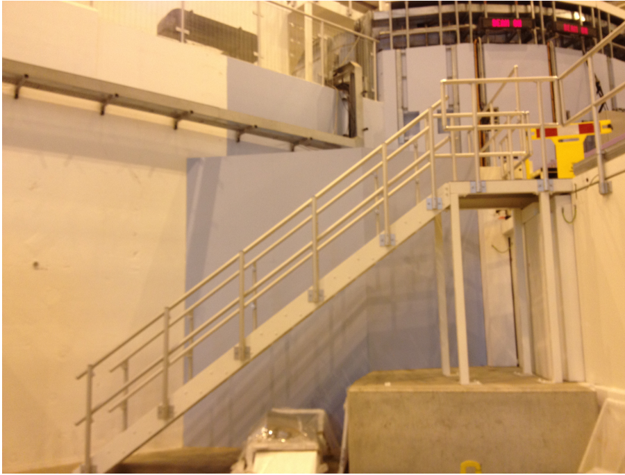
Figure 2: Fully grouted shielding walls at ISIS, with no obvious gaps between the permanent structures. The gaps are sealed at the rear, then the cement is pushed into the gap and smoothed flat.
