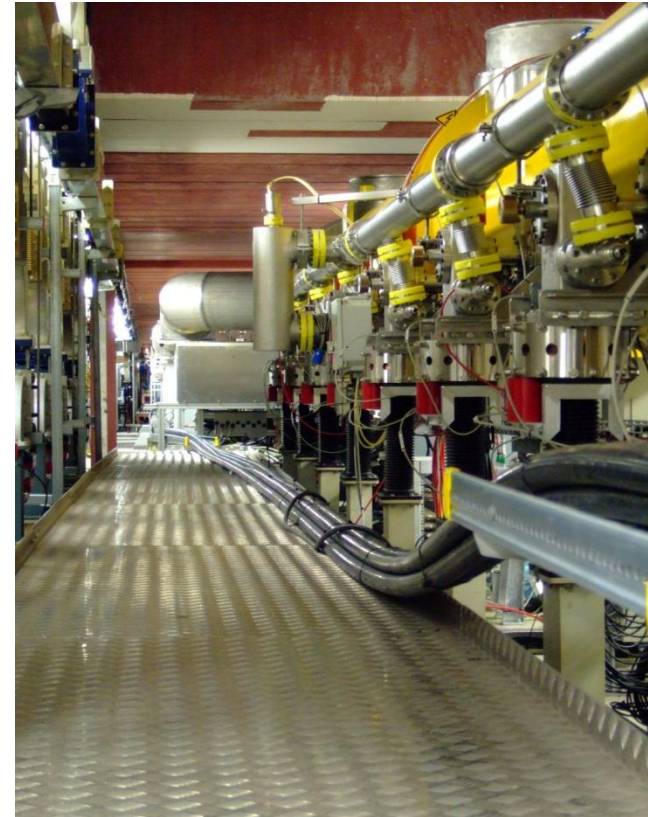
Cables behind ACC module
