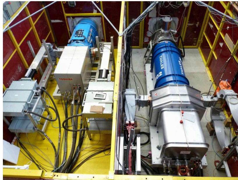
Horizontal multibeam klystron prototypes at the klystron test facility (KTF)
