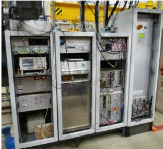
Modulator control racks
