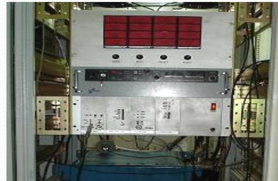
Interlock, control and trigger chassis.
