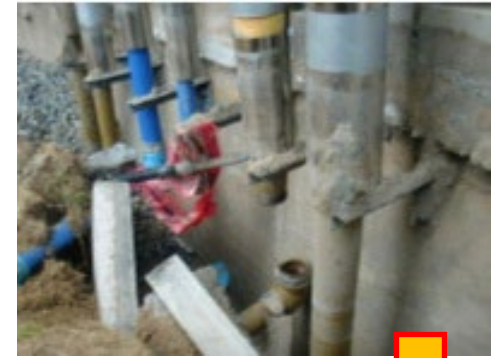
Water/gas pipes broken
