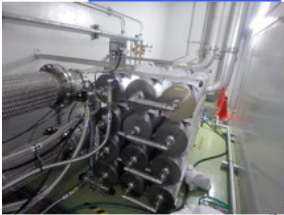
He-gas collection tank (main)
