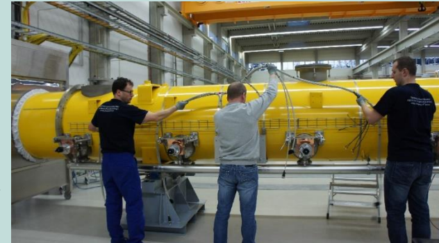
Cabling of the cryomodule
