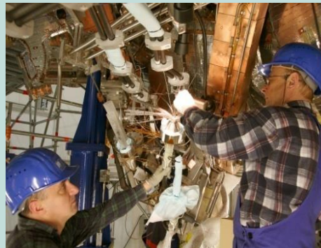
Electrical connection of the coil current leads and bus bars
