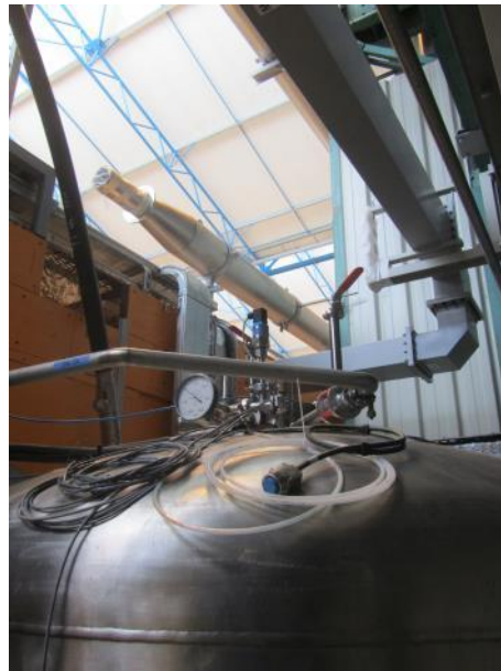
Cryo plant distribution (ready)
