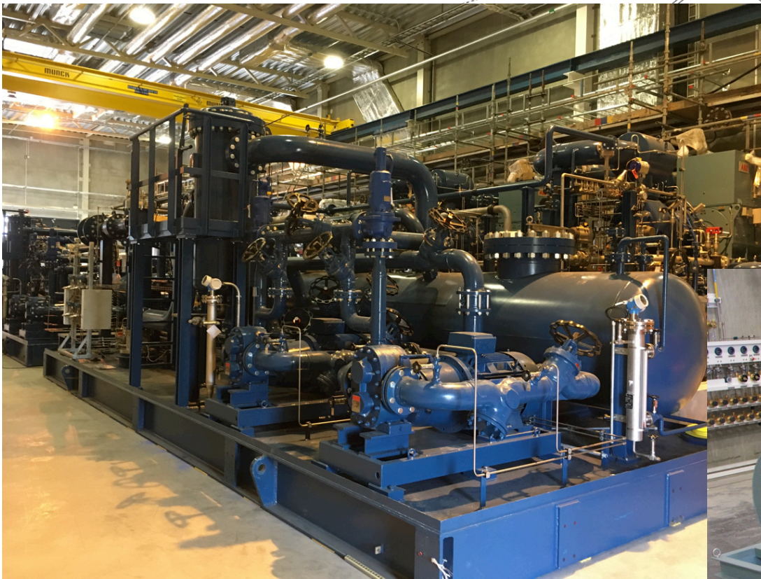
ACCP compressors and oil removal system
