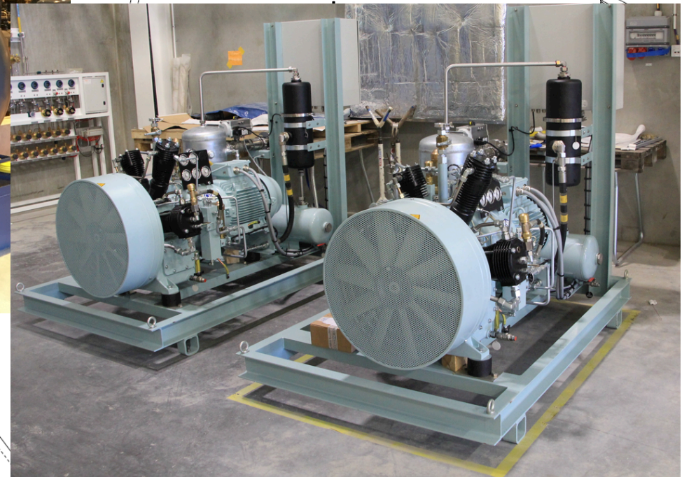
Helium Recovery System Compressors
