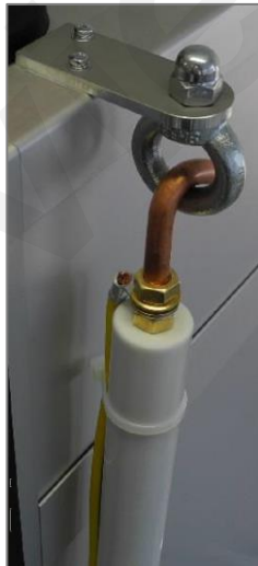
Figure 9: Grounding rod connection to HV platform
