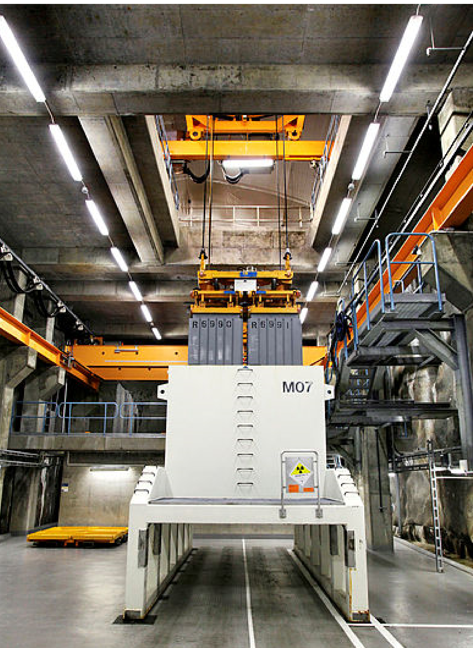
24/29 Loading of moulds from ATB 12K into a silo
